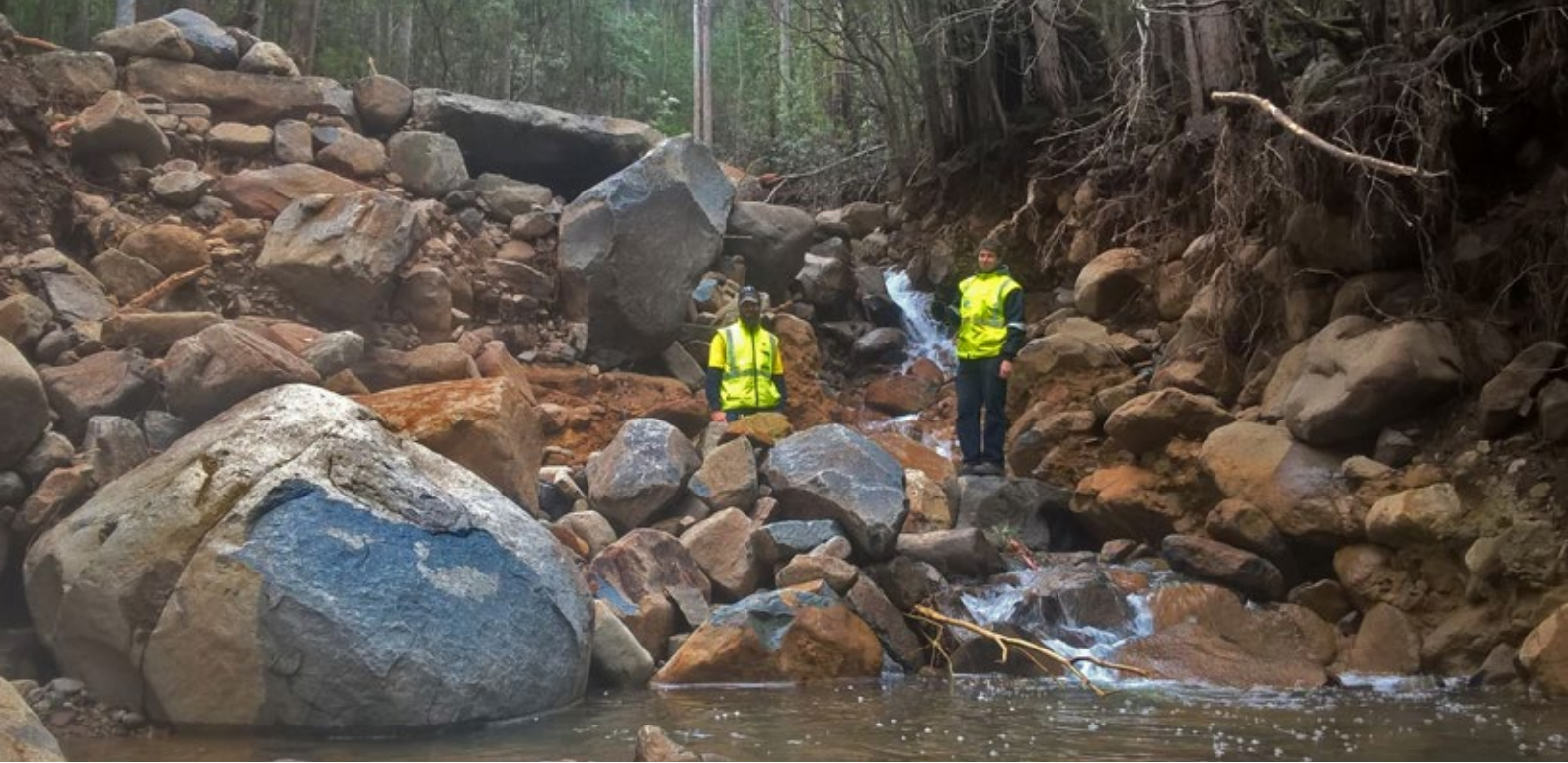
North-South Track – staff assessing damage at the Clapper bridge.
